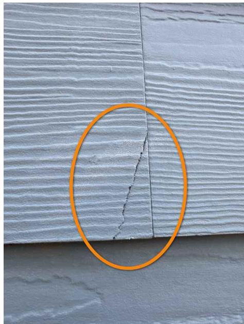
Additional photo of this finding showing the damaged siding.
