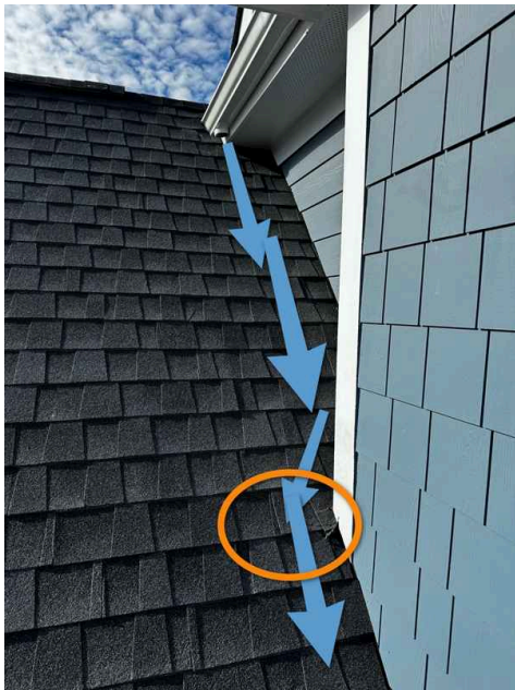
See description and following photos regarding the circled area. A larger amount of water flows past here.
