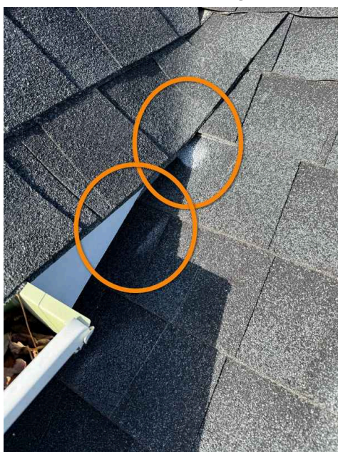
Additional photo of this finding.
