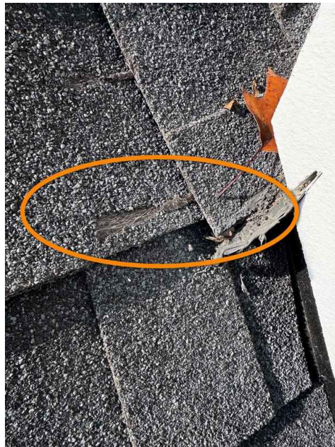
This shingle is completely damaged. Replacement is needed.
