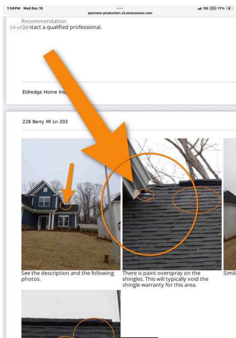
This finding was described in a previous report. Repairs have not been made in this area.
