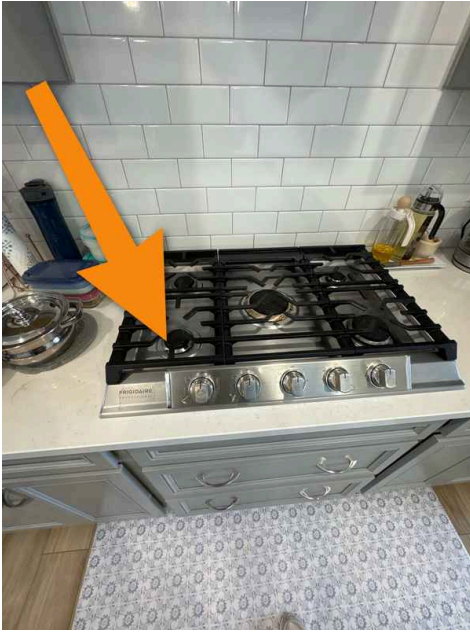
This burner does not light consistently.
