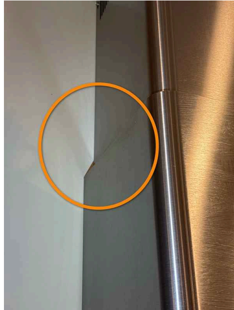
Additional photo of this finding.
