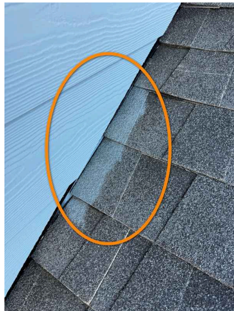
Additional photo of this finding.
