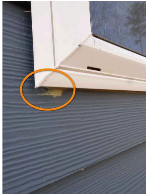
Additional photo of this finding showing missing paint.
