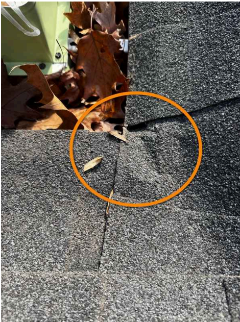
Additional photo of this finding showing that the shingle is creased and damaged.
