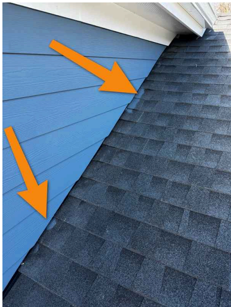
See description and following photos. Paint was found on the shingles.
