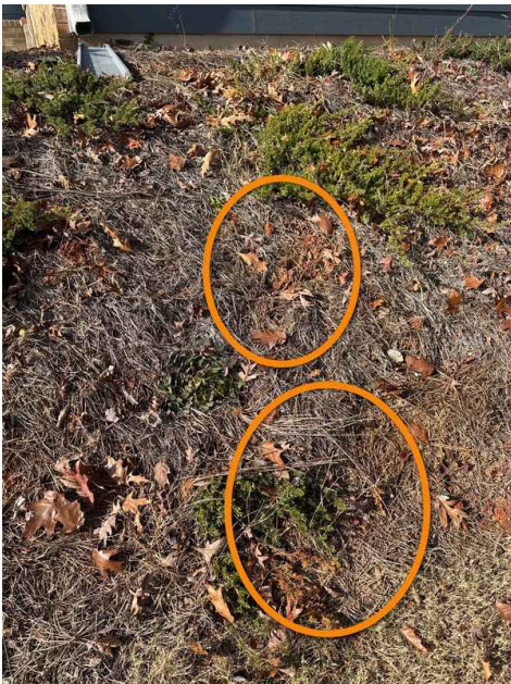
Additional photo of this finding under the pine straw.
