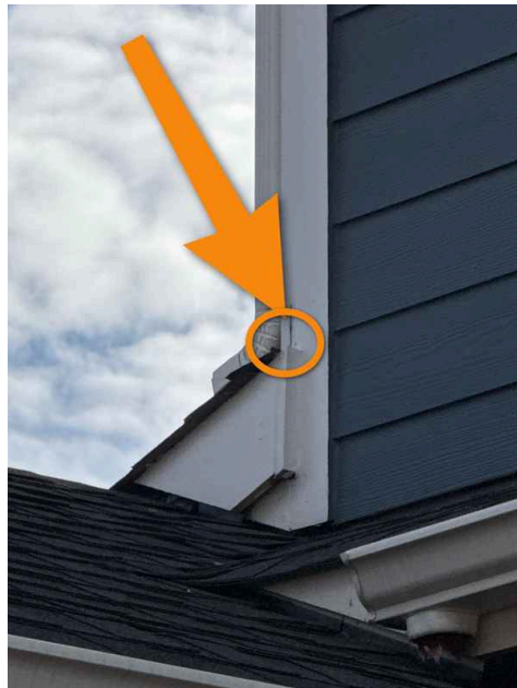
Additional photo of this finding.
