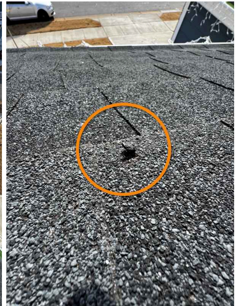
Additional photo showing that a raised nail has punctured the shingle.
