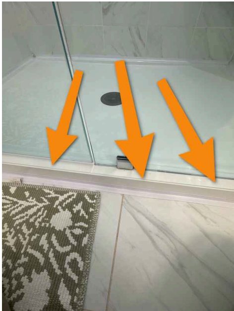
This means that excessive amount of water spill out just outside the shower here.
