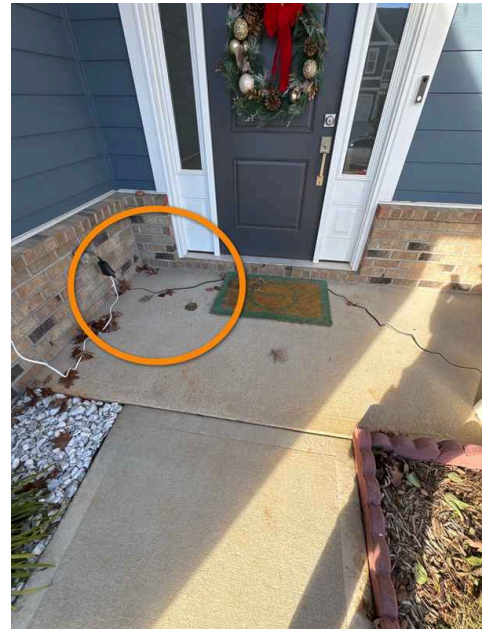
See description for this finding. Water collects in the circled area when wind driven rain hits the porch.
