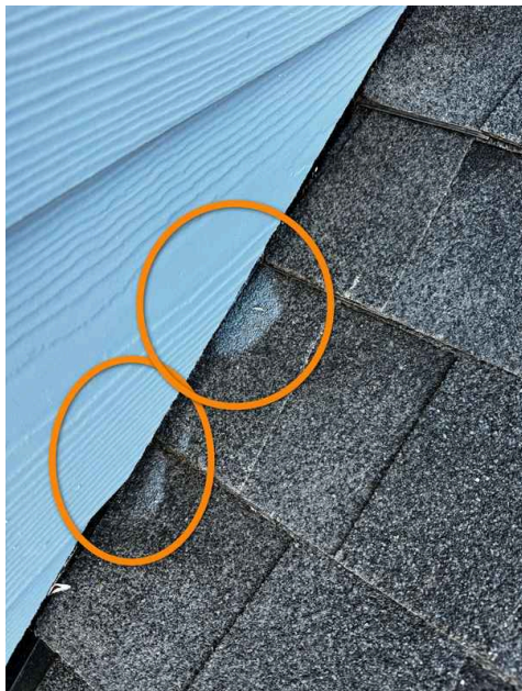
Additional photo of this finding.
