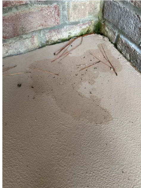
Additional photo of water on the porch from the leak.
