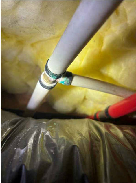
This fitting is corroded.
