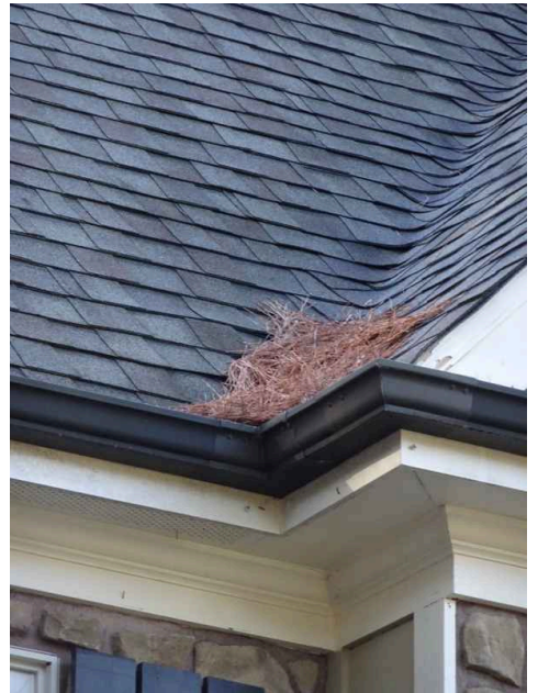
See description for this finding.
