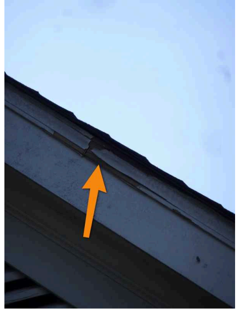
See description for this finding.
