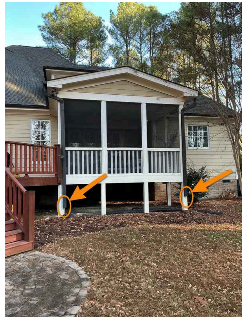
Location of the following findings at the rear deck.
