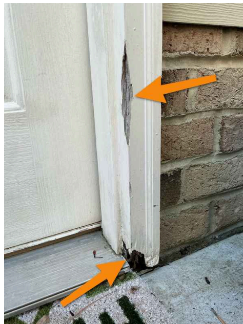
See description for this finding.
