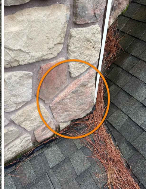
This stone is slightly loose which is typical of hidden damage.
