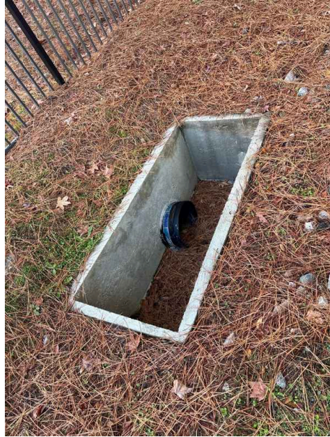
This presents a trip/fall hazard. See description for this finding.
