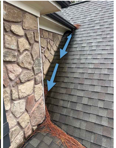
Too much water is directed against the stonework here. Hidden damage is expected.
