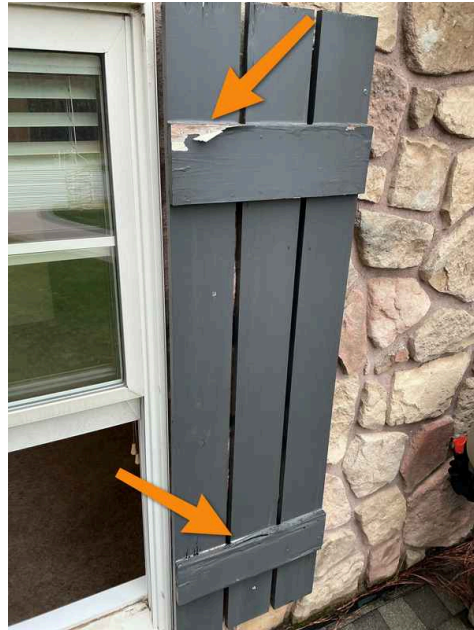
See description for this finding.
