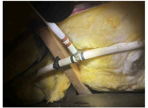
This fitting is corroded.
