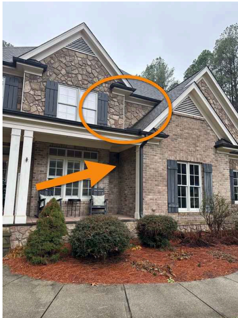
This area is leaking to the wall below.
