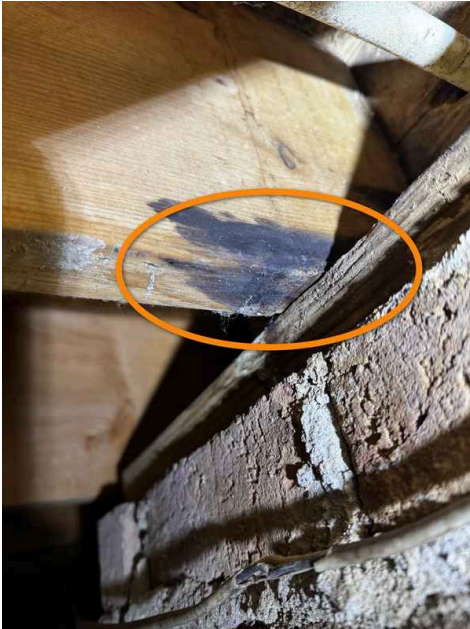
Additional photo of this finding showing that the damage is also beginning to decay the floor structure.
