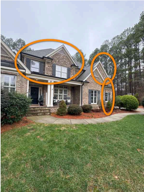
See description and following photos. Damage was found in the crawlspace caused by leakage from above the porch. This means hidden damage in the walls at each end of the porch is expected.
