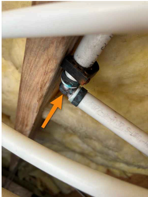
See description for this finding.
