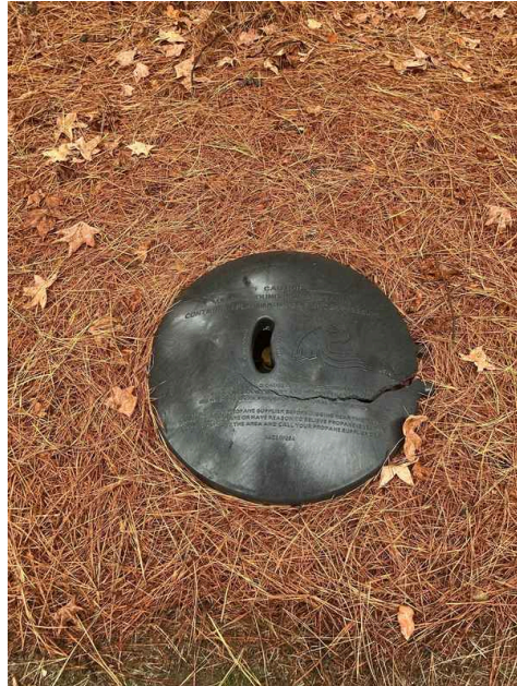
See description for this finding.
