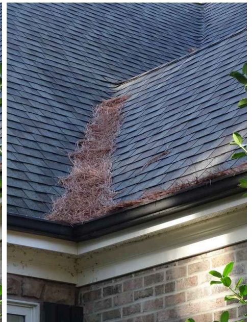
See description for this finding.
