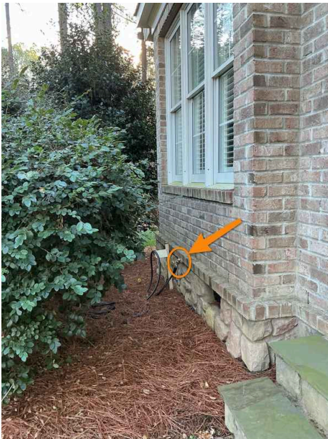
Location of the following finding at the front of the home.
