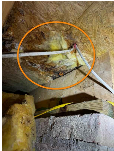
The subfloor is decayed here at the rear left corner of the front porch. This means that hidden damage is expected in the wall above this area.
