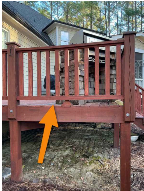
The deck structure was noted to be sagging slightly due to the excess weight of the stone Grill stand. See description for this finding.
