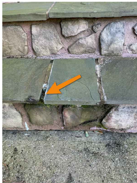
Mortar is missing inbetween the stone surface which allows the water to cause the steps to come loose.
