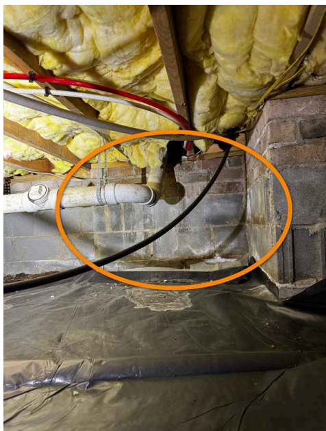
The foundation wall is wet here between the garage and front porch area. Significant amount of water flow down the wall from the roof above the porch. See following photos.
