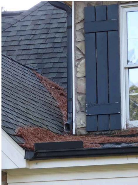
See description for this finding.
