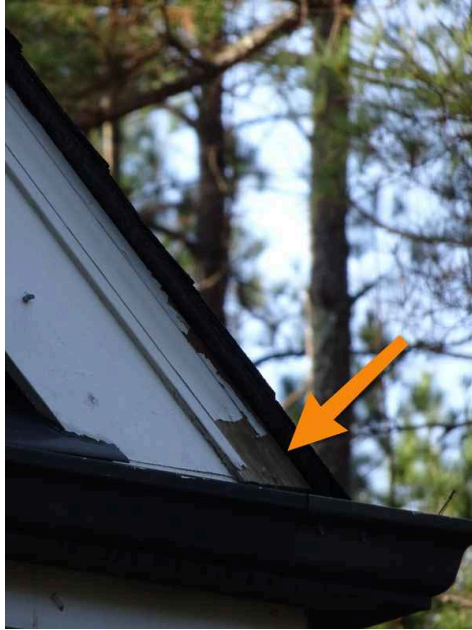
See description for this finding.
