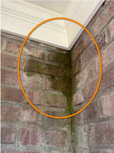
Additional photo of this finding showing the wet area of brick.
