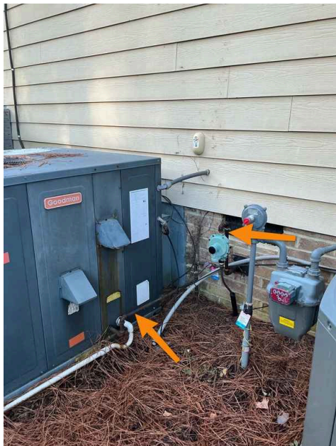
Location of the following finding at the exterior package unit.
