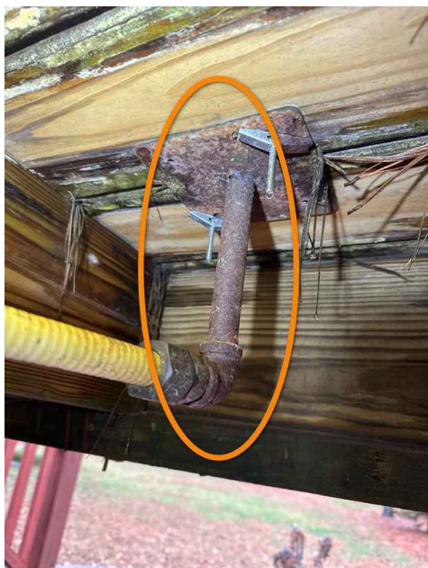
Additional photo of this finding located under the gas grill.
