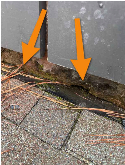
Moss buildup on the stonework indicate excessive moisture caused by improper installation.
