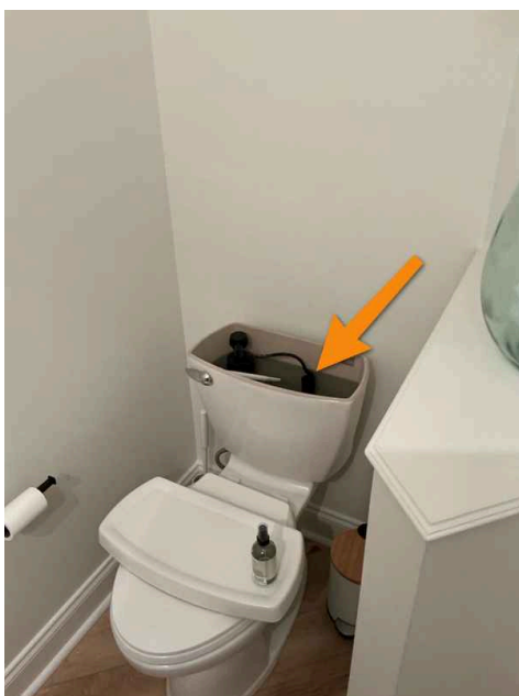
Location of the following finding in the downstairs bathroom.
