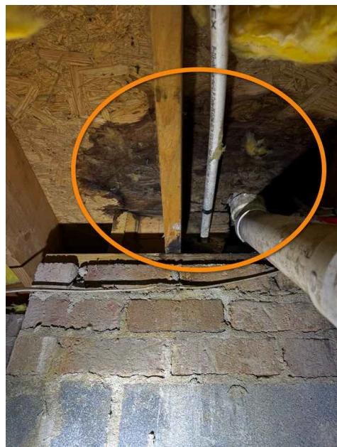
Additional photo of this finding behind the wall to the garage/front porch.
