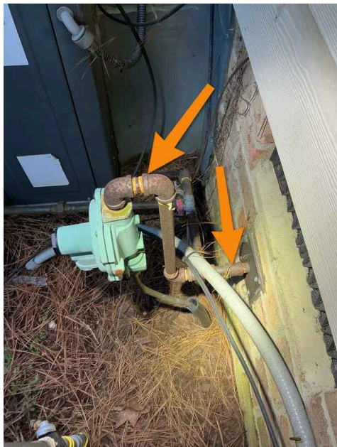
The gas line is rusty and corroded.
