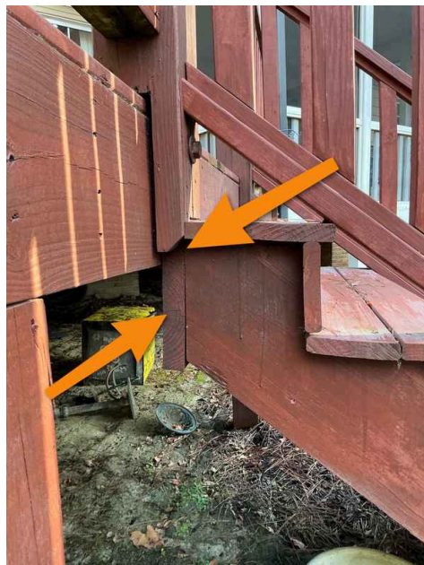
The deck stair stringers are tip loaded making them unsafe for future use.
