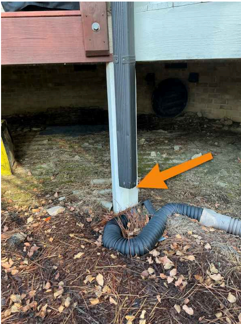
The downspout elbow/extension is missing here.
