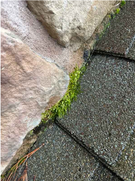
Moss growth indicates frequent excessive moisture.
