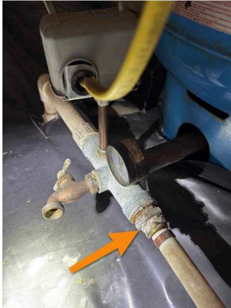
This fitting is corroded.
