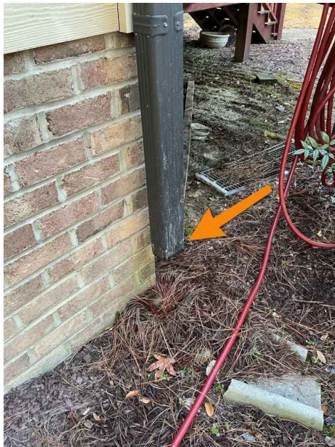
This gutter is missing the downspout elbow and extension.
