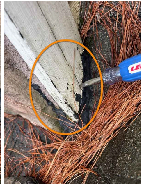
Additional photo of this finding showing the decay.
