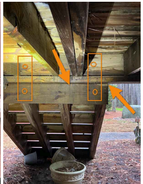
More lumber and bolting is necessary on the back of the stair stringers. See description and following photos.
