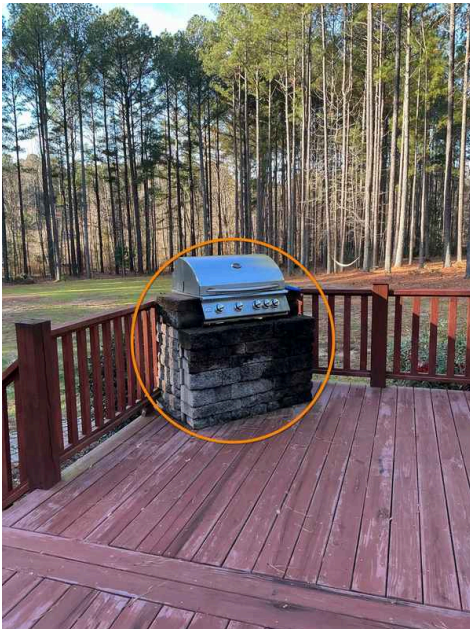
The deck structure is not rated for this amount of weight. See description for this finding.
