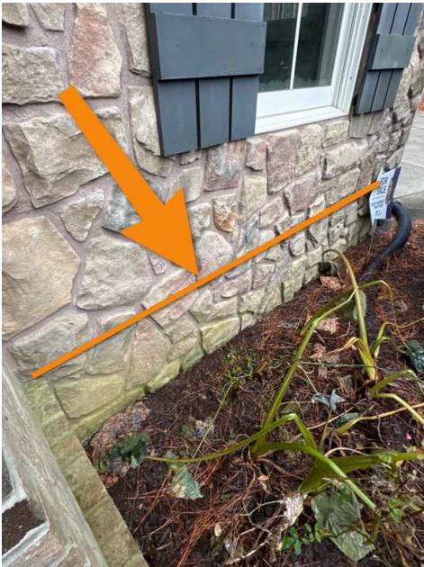
There is no weep system where the wood structure of the home begins.
