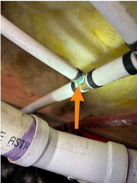
Other corroded fittings were noted in the crawlspace.
