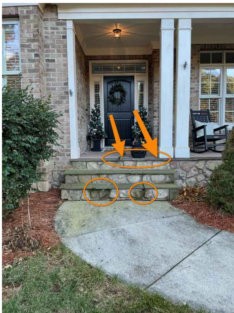
Location of the following finding. The two stones at the top are loose.
