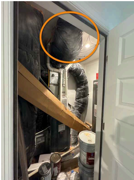
Insulation falls from the attic when the doors opened. This means the fire blocking between floors is missing.
