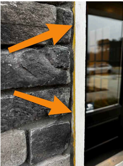
Similar findings were found here where there is no transition strip. Also, the trim is not painted which means it does not protected.
