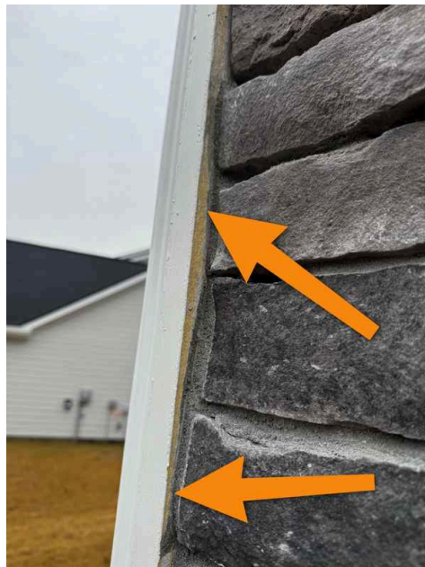
This unpainted trim is not projected by a transition strip and is not painted. This area is exposed to water each time it rains.
