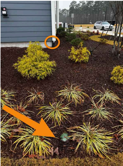
See description and following photos. Water overflows in the circled area by the home.
