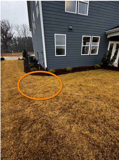
The pop-up cap for this downspout could not be located. This cap is likely covered with grass.
