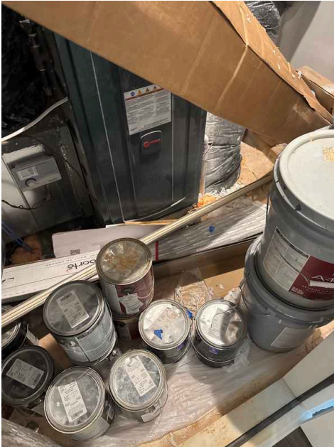
The utility room is excessively dirty. All areas should be cleaned.
