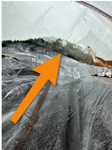
Additional photo of this finding looking up at the ceiling showing some of the gaps.
