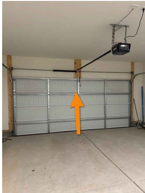
Also, the spring/springs should be adjusted. The door is difficult to raise by hand.
