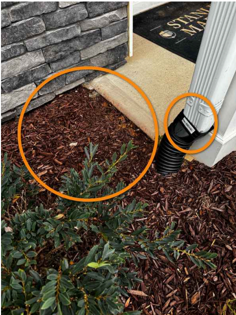
The mulch is being washed away because water overflows from the downspout.
