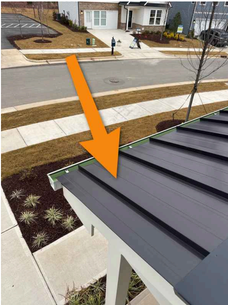
See description and following photo. The roofing is damaged from material such as a raised nail that was under the roofing..
