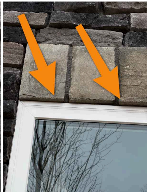
Additional photo of this finding, there is no weep system above the windows. The area above the windows and garage door are the most likely to become decayed.
