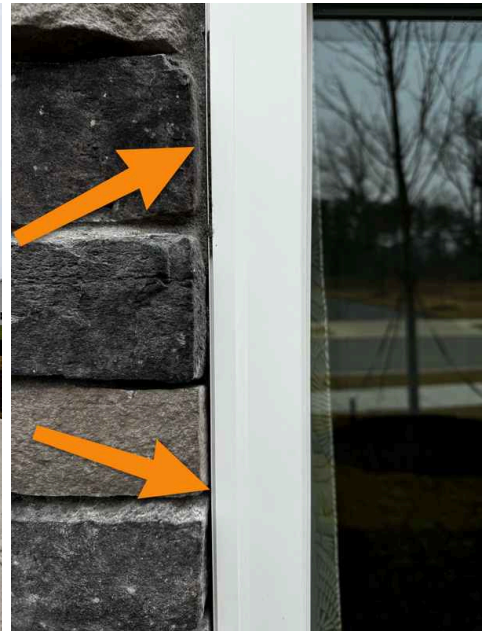
There is no transition strip between materials.
