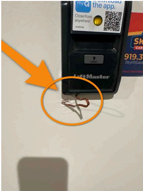
The wiring below the button is visible.
