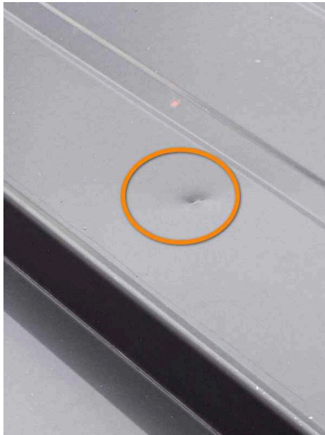
This raised nail may puncture the Roofing at any time.
